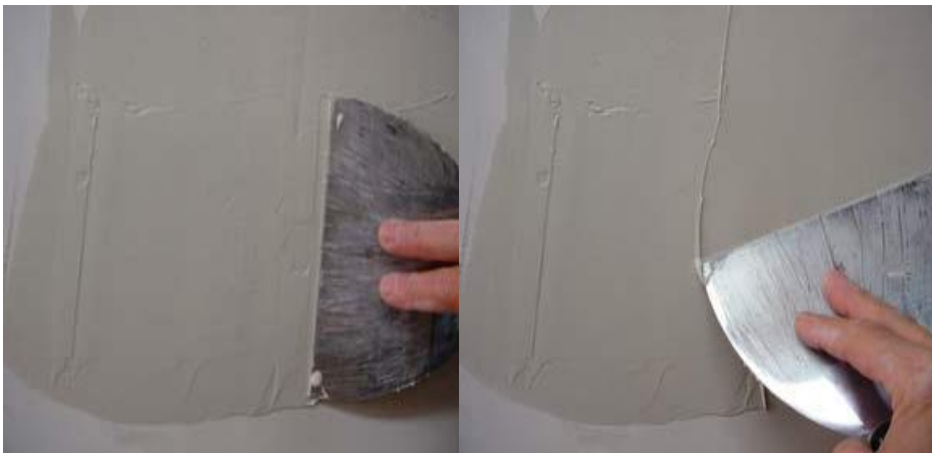
Figure 5 .2 cover the joint damage joint
